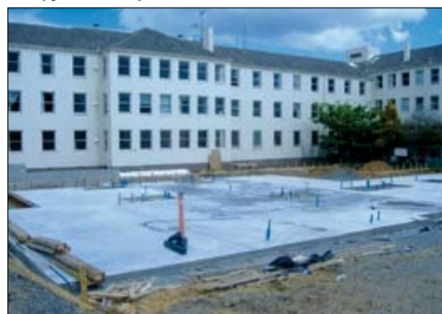
BELOW: When complete in November 2008, this new Inpatient Centre will occupy all the hospital wards and the HDU.
