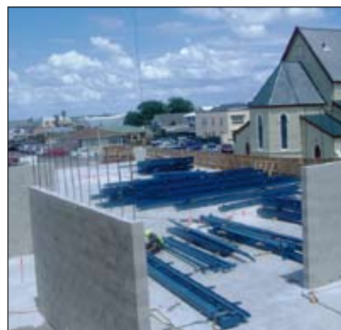
ABOVE: The concrete has been laid for the new Thames Clinical Centre and construction is expected to be complete in August 2008.
