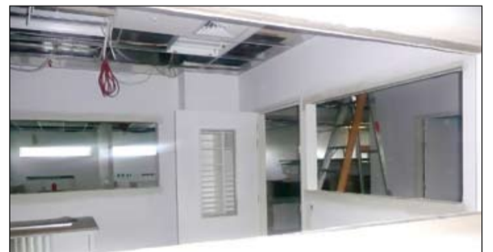
PEEK INSIDE: The inside of the Thames Clinical Centre are starting to form and work is to be complete by September.
