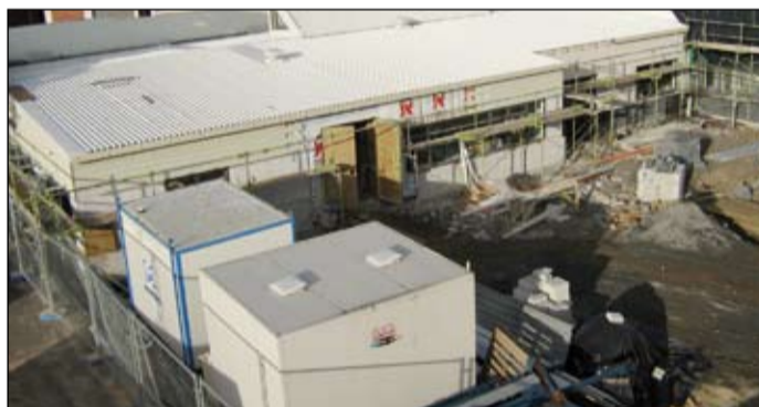
LINKED: The Inpatient Centre is being built in three stages with the third connecting to the new clinical centre.
