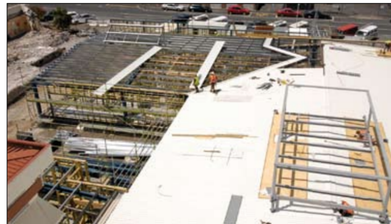
MAKING PROGRESS: The TCC roof will be complete by the end of the month.
