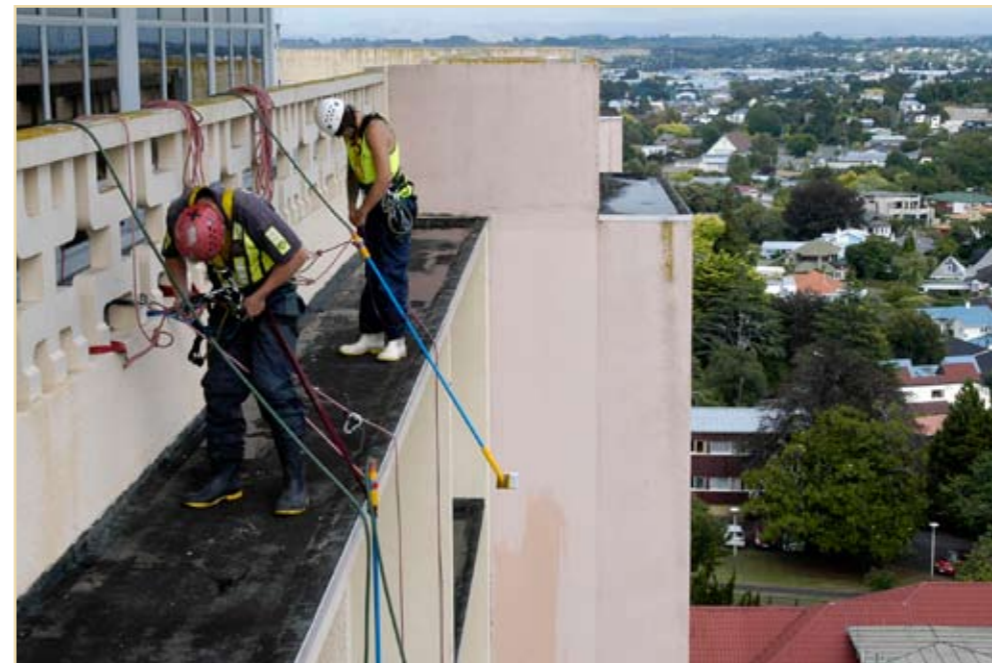
HIGH SIGHTS: These workers had a great view last month when they abseiled down the Menzies Building to clean the windows on a clear Hamilton morning.
