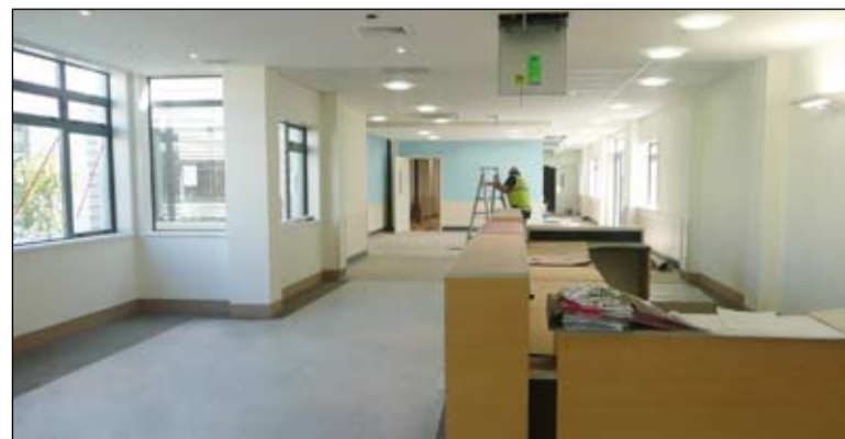
FINISHING TOUCHES: The clinical centre interior is nearing completion as everything is checked and finalised. Including the emergency department assessment bay (top) and outpatients reception (bottom).
